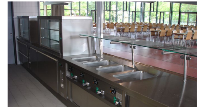
Hot service counter
